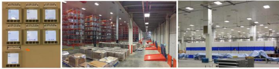
Figure 4. Digital power meter for lighting, power, process, mechanical equipment, and flexible lighting controls to optimize energy savings.
