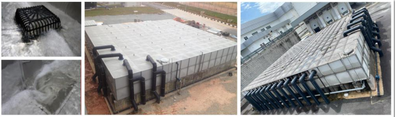
Figure 9. Syfonic gutter and Rain Water Downpipe System with North and South rainwater harvesting tank
