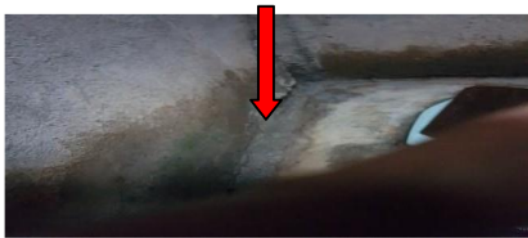
Figure 8. The floor of the 3 rd house cracked(Source: Author document)
