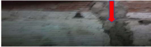
Figure 6. The wall of the 2 nd house cracked, covered with plaster(Source: Author document)
