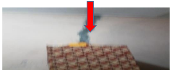
Figure 3. Cracked wall of the 1st resident's house ( Source: Author document)
