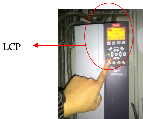
a. Local Control Panel
