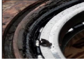
Fig 8. Deformed floating seal is damaged
