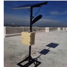
Gambar 3. 14 PJUTS solar Tracking
