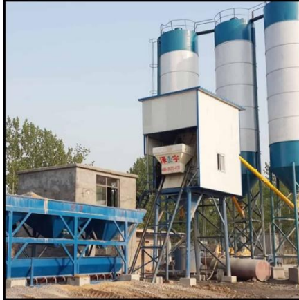
Gambar 4.25 Wet Mix Storage Silo
