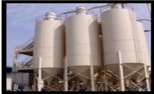
Gambar 4.15 Batching Plant Dry Mix Plants
