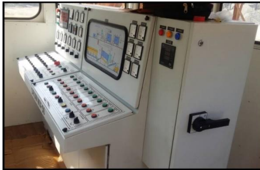
Gambar 4.24 Control Cabin Unit
