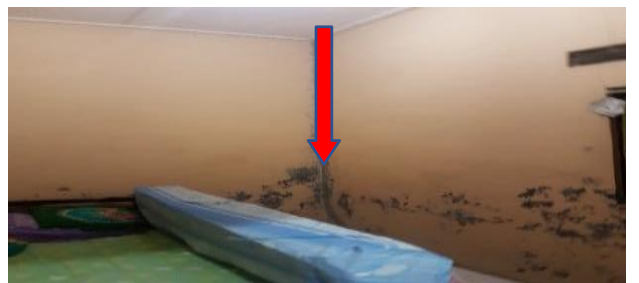
Figure 5. Wall-cracked restroom of the 1 st resident's house (Source: Author document)
